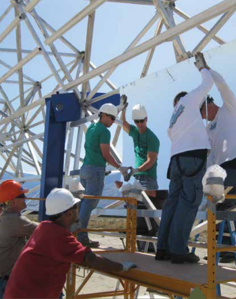
Technicians mount mirrors as part of the College of the Desert's Utility-Scale Solar Energy Program.
