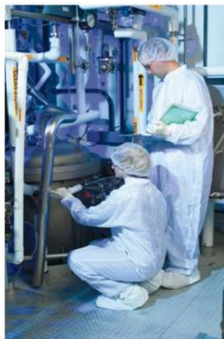
Figure 1-16. Validation technicians locate temperature probes in a process using drawings called Piping & Instrumentation Diagrams (P&IDs)
